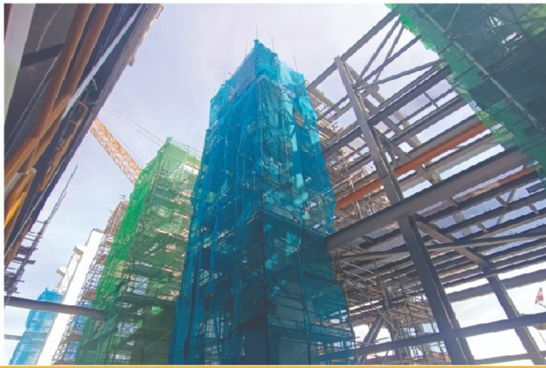
23 Gul Avenue Project Project Location - 23 Gul Avenue Project Ref No: - A1982-00009-2016 Our Client JMJ Consultants Pte Ltd
