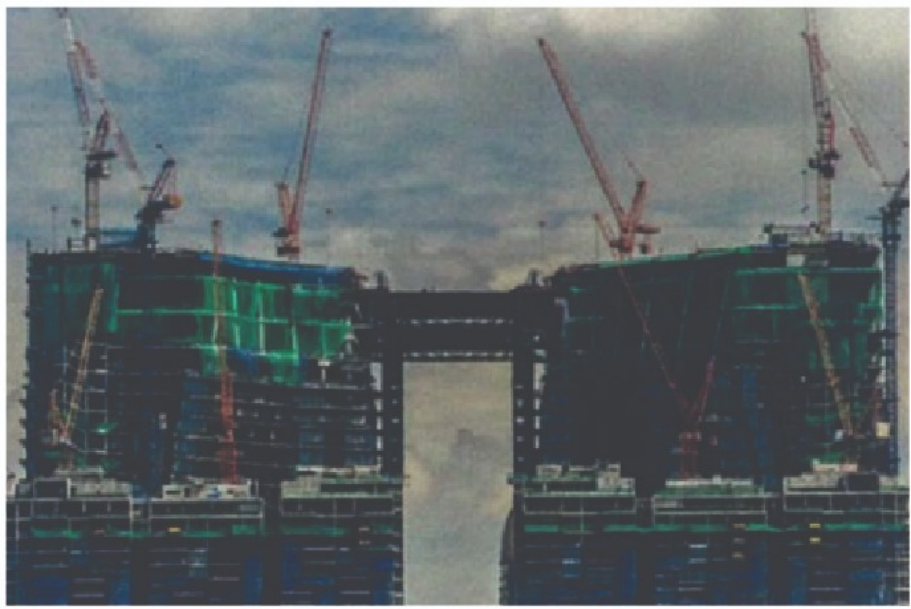
Marina One Hyundai GS Project Marina one mixed development project at Central Boulevard Singapore.
